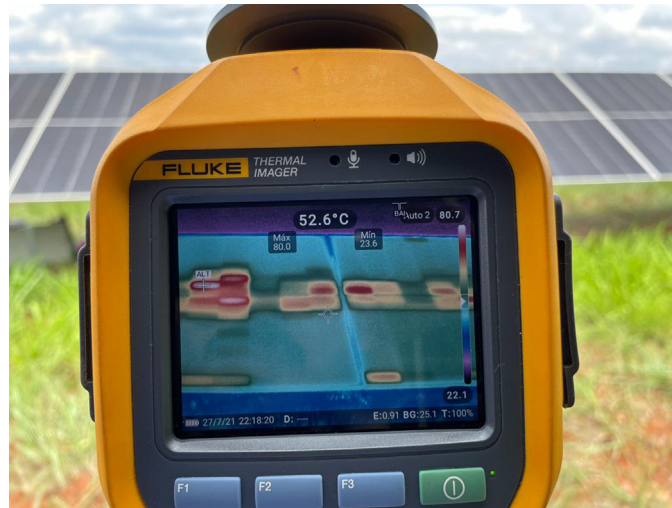
Fig. 12. Thermography of PV modules using the Fluke Ti450 infrared camera.
