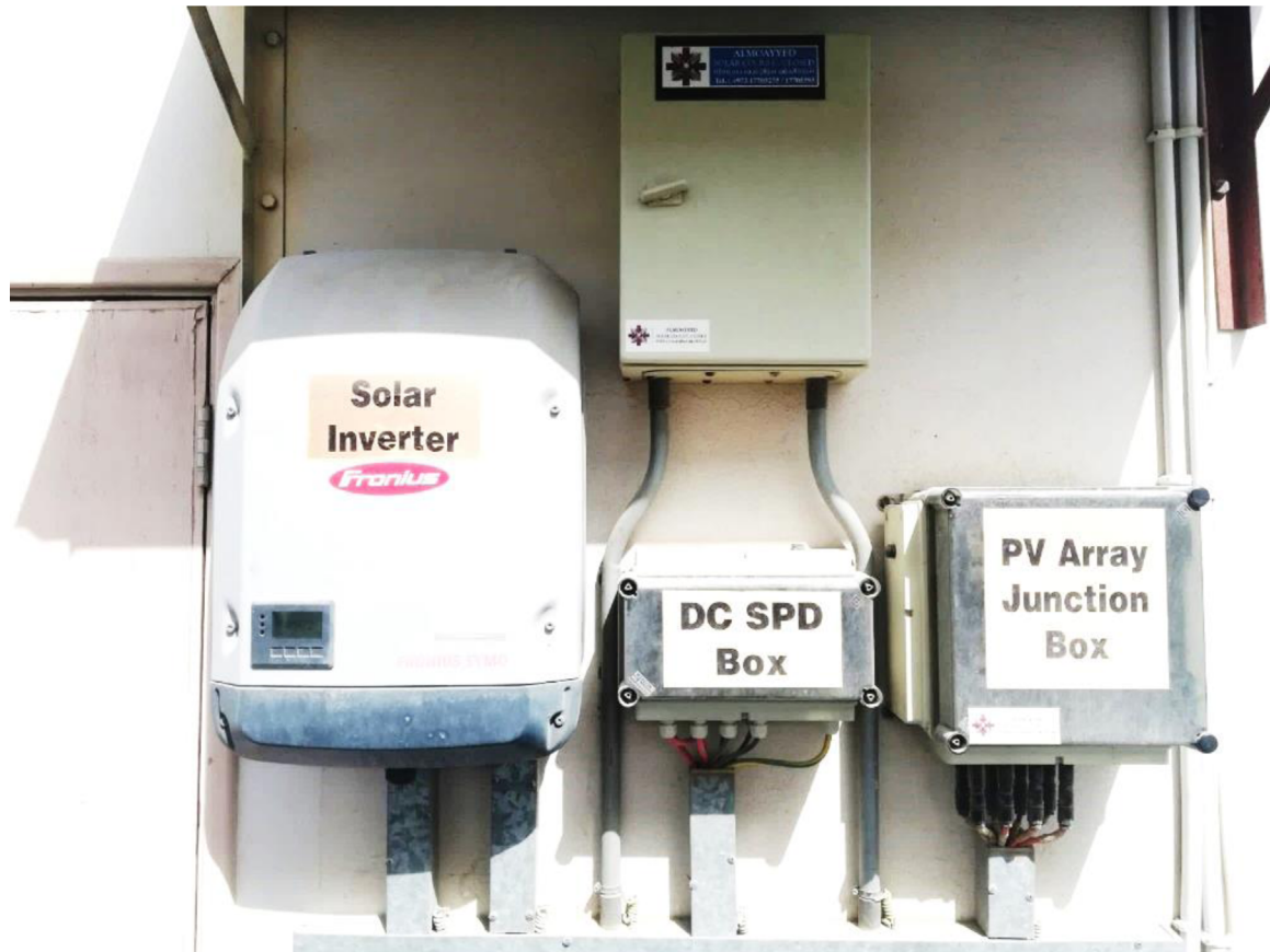
Fig. 3. The main components of PV power electronic systems for PV array installed at all 7.8 kW – PV domestic buildings (houses # 1 to #4) in Bahrain. These components are Smart PV meter, PV array junction box, DC SPD box and solar inverter.
